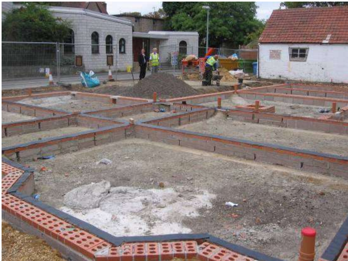
Work has begun on the new Student Accommodation. (This picture was taken from Benson Place, looking towards Resurrection Church)
